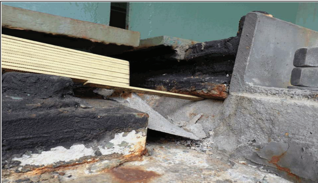
32 PIER 4, SPAN 5, BEARING PEDESTAL 5 SOUTH SIDE - FAILED REPAIR WITH BEARING LOSS
