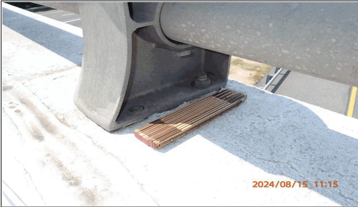
13 SPAN 4, WEST METAL RAIL AT POST 4 - SHEARED ANCHOR BOLT AND MISSING NUT
