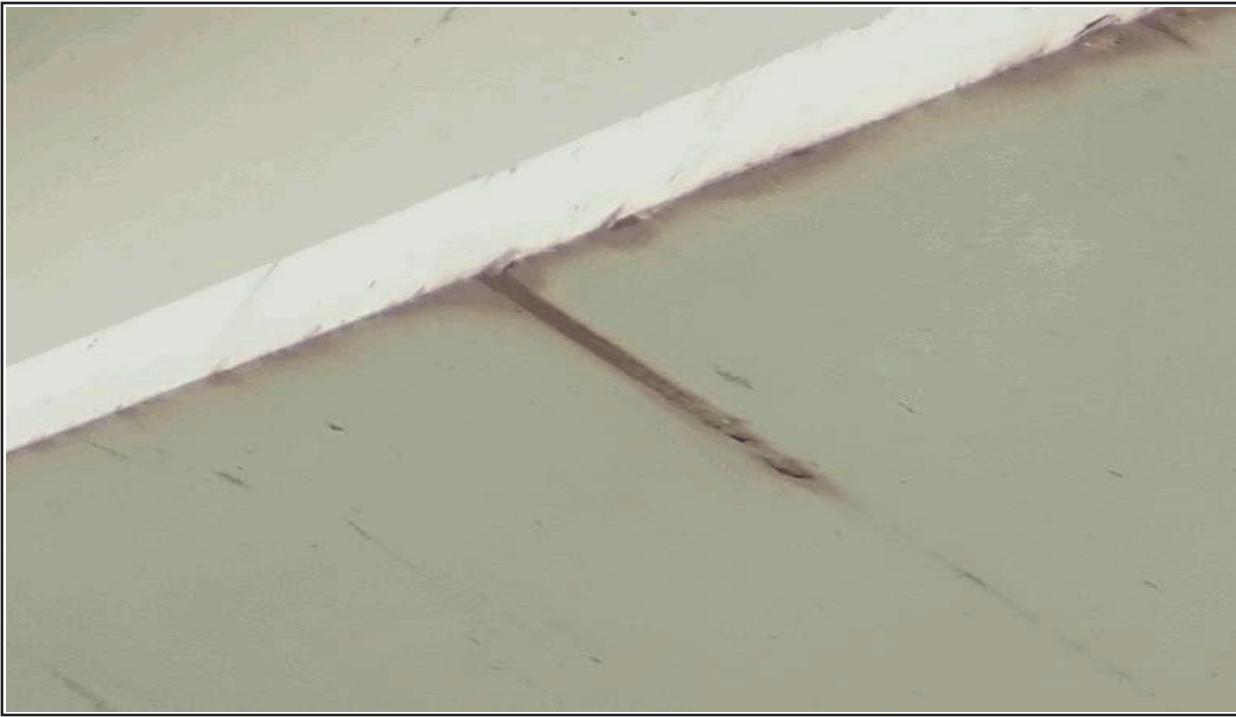
23 SPAN 4, GIRDER 5 OVER RIGHT LANE - TRAFFIC IMPACT GOUGE AND SCRAPE
