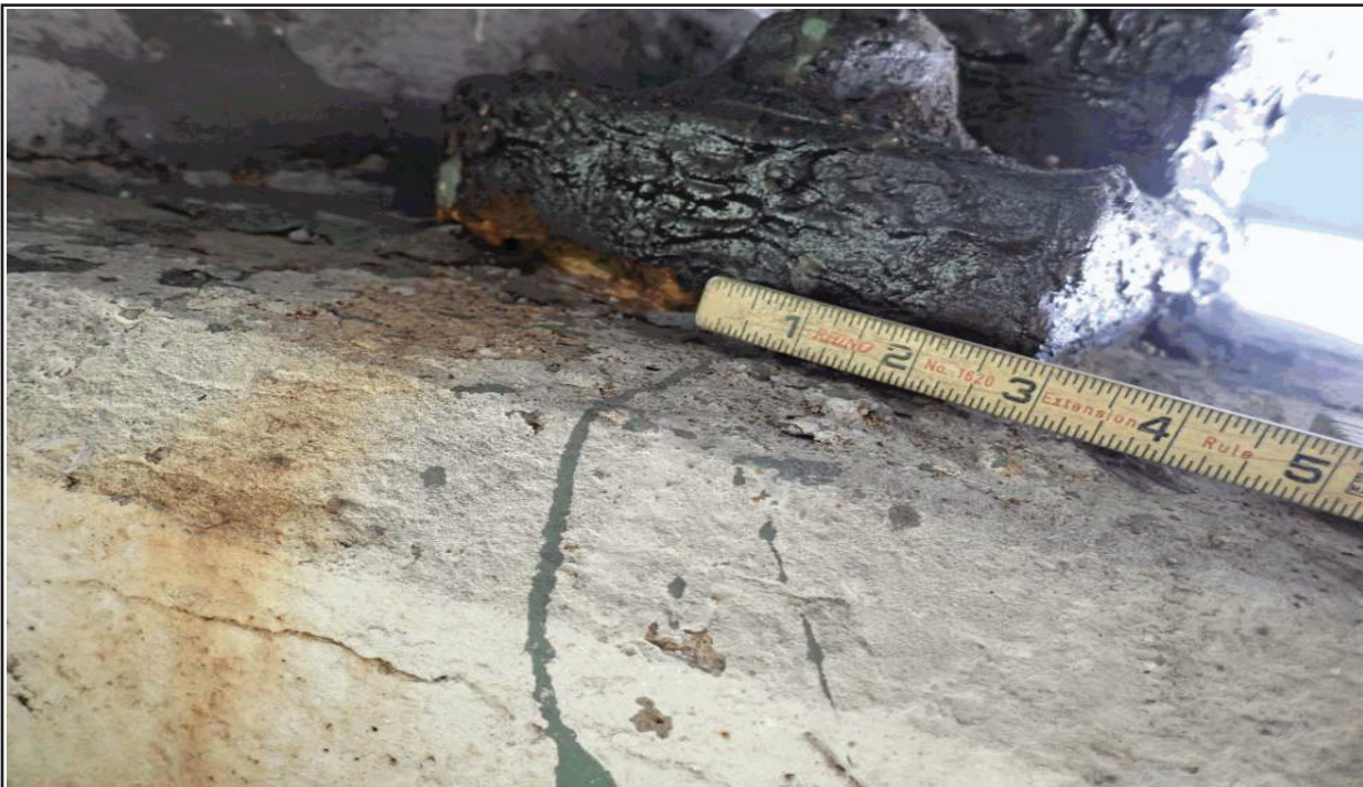
30 PIER 4, SPAN 4, BEARING 4 - LAMINAR CORROSION WITH SECTION LOSS ALONG THE MASONRY PLATE
