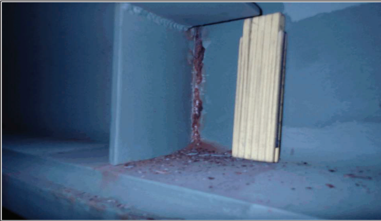
25 SPAN 4, BAY 4 AT GIRDER 4 WEB STIFFENER TO DIAPHRAGM 2 - CORROSION ALONG WELD (NO CRACK FOUND)
