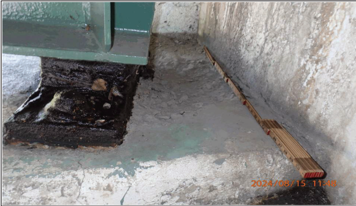
35 SOUTH ABUTMENT, BEARING PEDESTAL 5 - PAINTED OVER SPALL BEHIND BEARING
