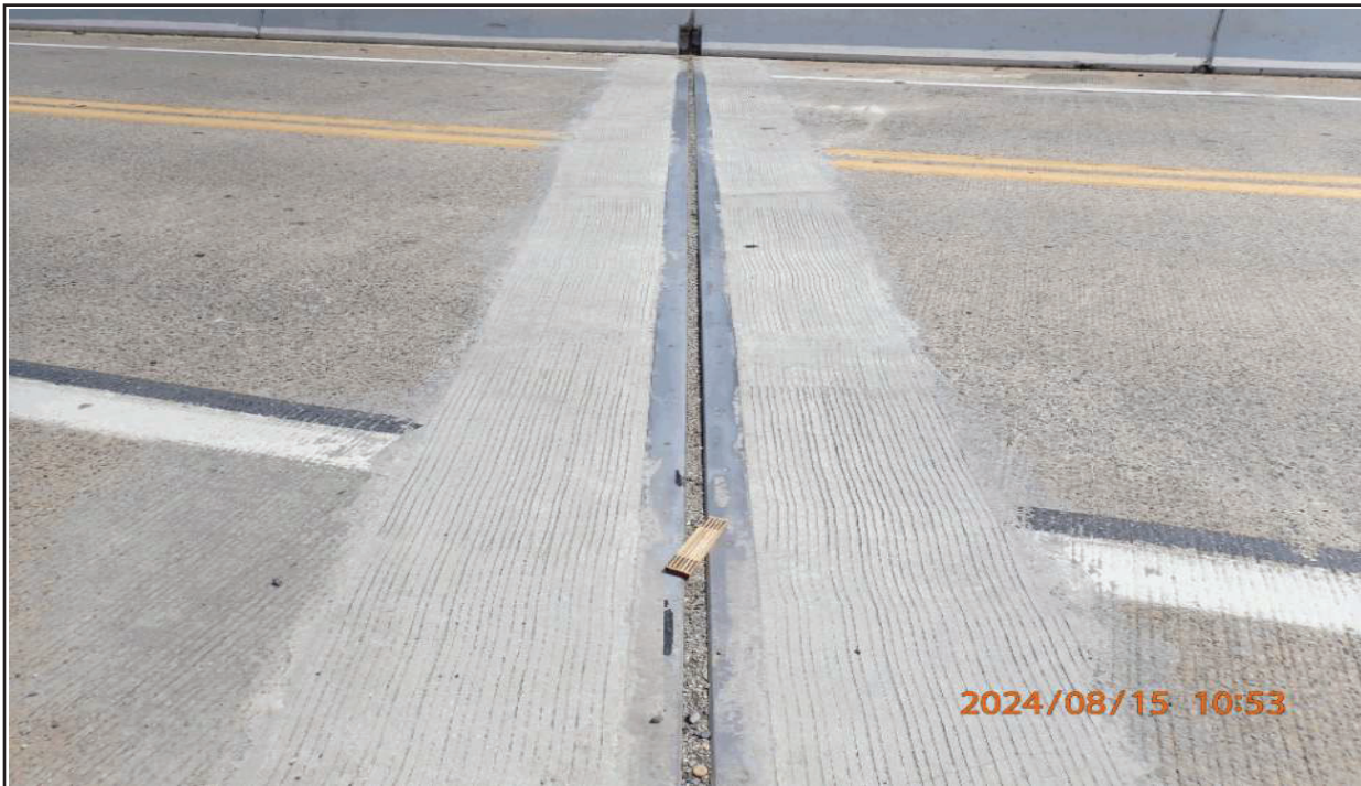
10 SPAN 3 STRIP SEAL JOINT - FULL OF DEBRIS
