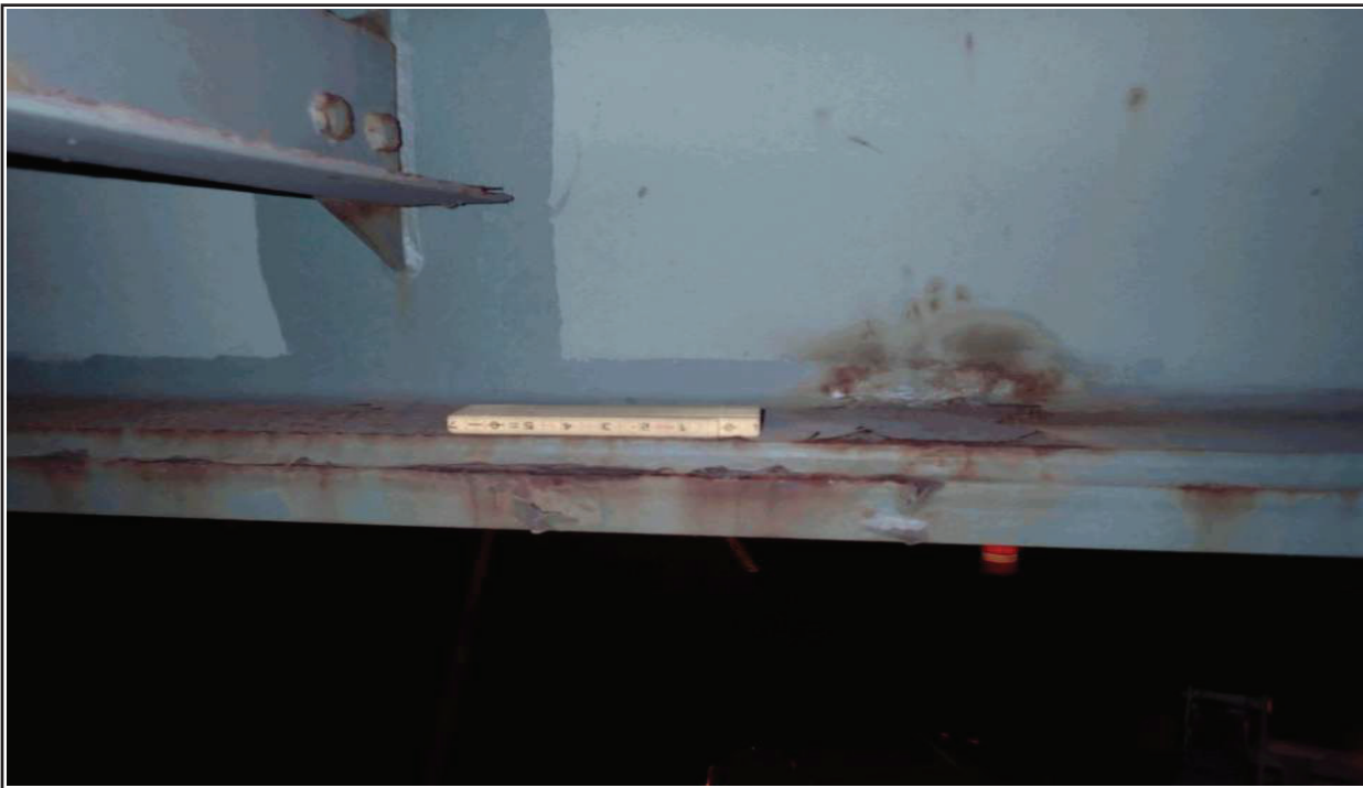
24 SPAN 4, GIRDER 4, BETWEEN DIAPHRAGMS 1 AND 2 - CORROSION WITH SECTION LOSS TO EAST BOTTOM FLANGE AND BOTTOM OF WEB
