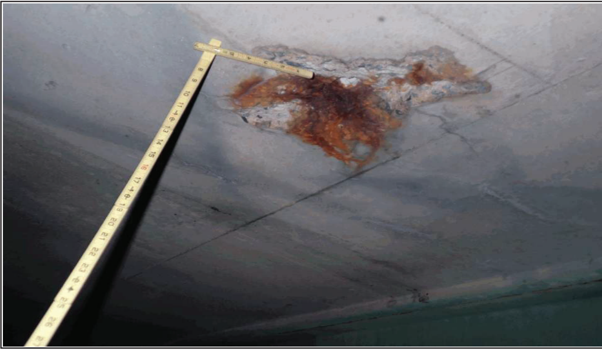
19 SOFFIT, SPAN 2, BAY 1 AT PIER 1 - SPALL WITH EXPOSED CORRODED STEEL REINFORCEMENT
