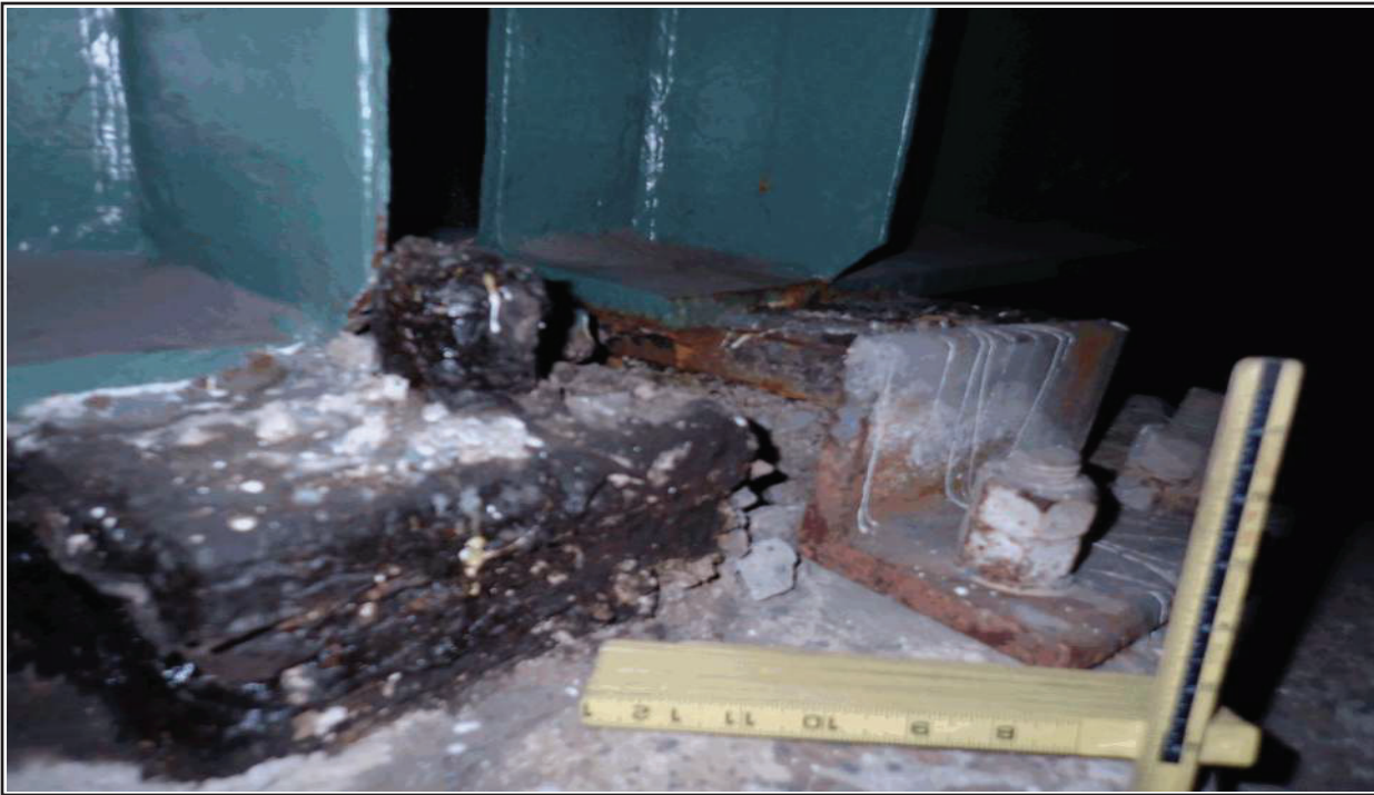
29 PIER 3, SPAN 3, BEARING 5 - VIEW OF KEEPER PLATE AND MISSING ANCHOR BOLT
