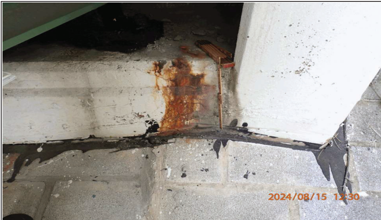
34 NORTH ABUTMENT, EAST END AT BEARING 5 - CRACKS WITH CORROSION STAINS
