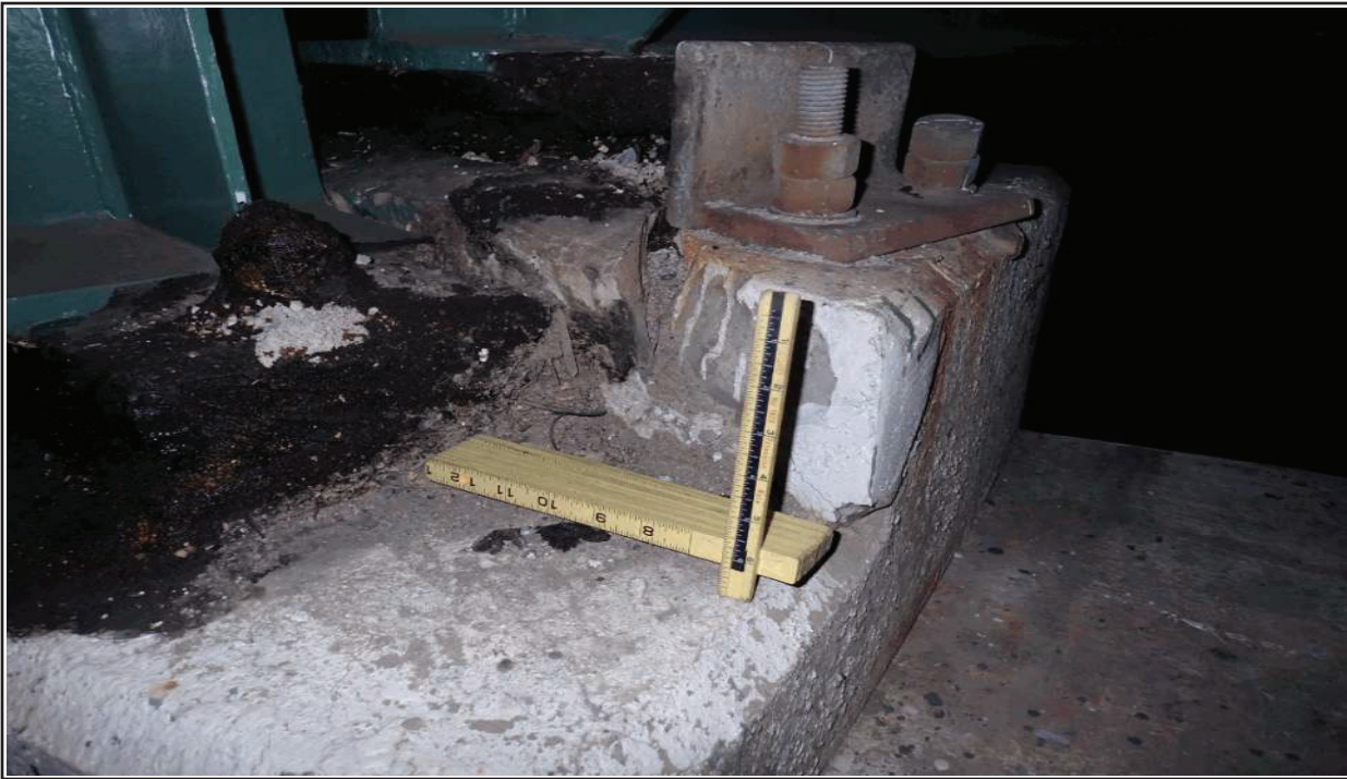
39 PIER 3, SPAN 3, PEDESTAL 3, NORTH FACE - SPALL / FRACTURE
