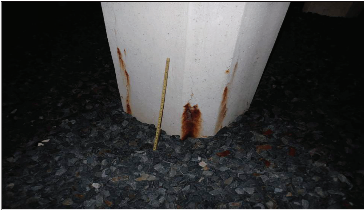
44 SPAN 3, PIER 3, COLUMN 3, NORTH AND EAST FACE - CRACKS WITH CORROSION
