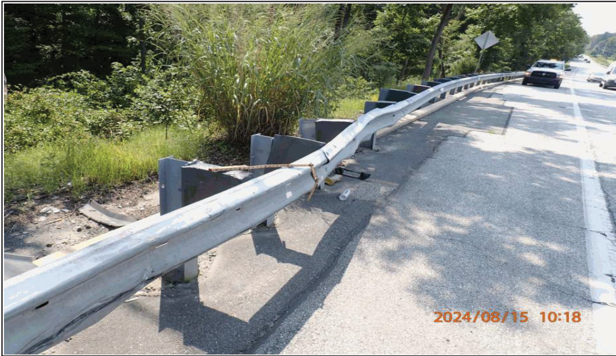
45 SOUTHEAST APPROACH GUARDRAIL - TRAFFIC IMPACT DAMAGE
