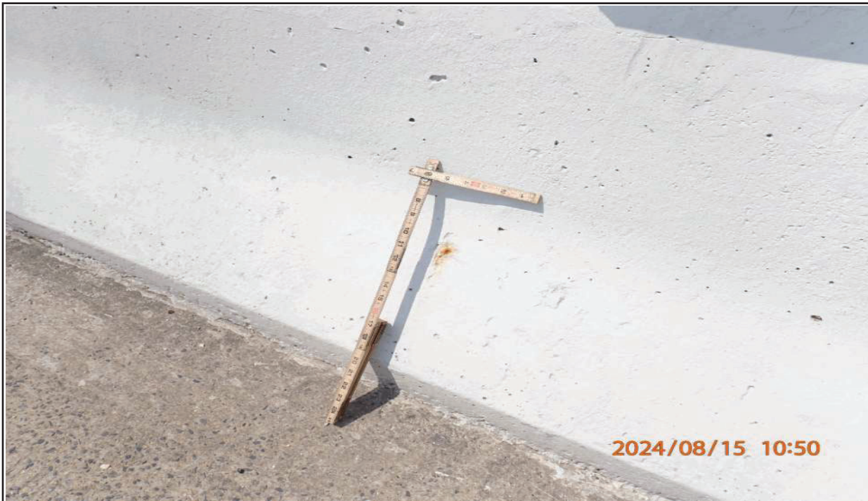
14 SPAN 2, WEST CONCRETE RAIL BETWEEN POSTS 7 AND 8 - EXPOSED CORRODED STEEL REINFORCEMENT WITH SECTION LOSS
