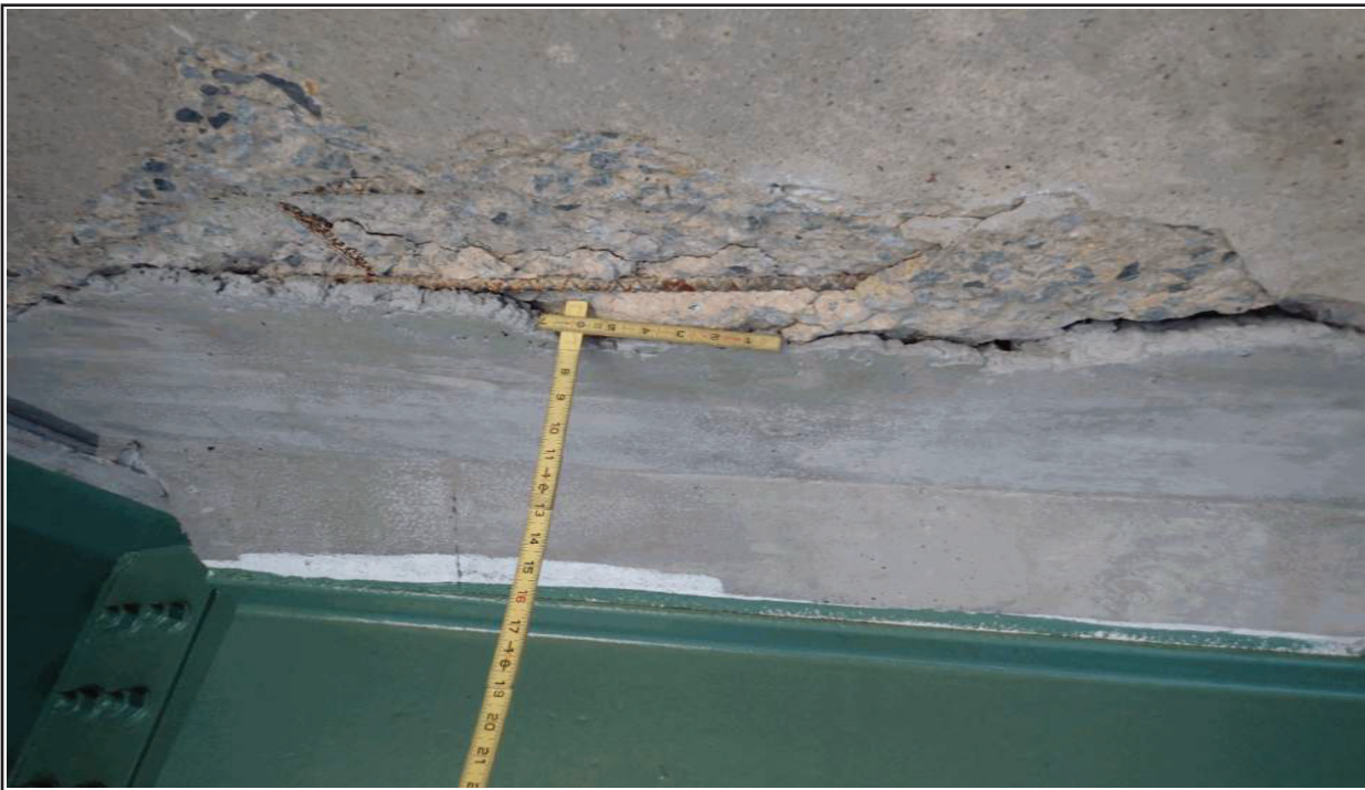
20 SOFFIT, SPAN 2, BAY 1 AT PIER 1 - SPALL WITH EXPOSED CORRODED STEEL REINFORCEMENT
