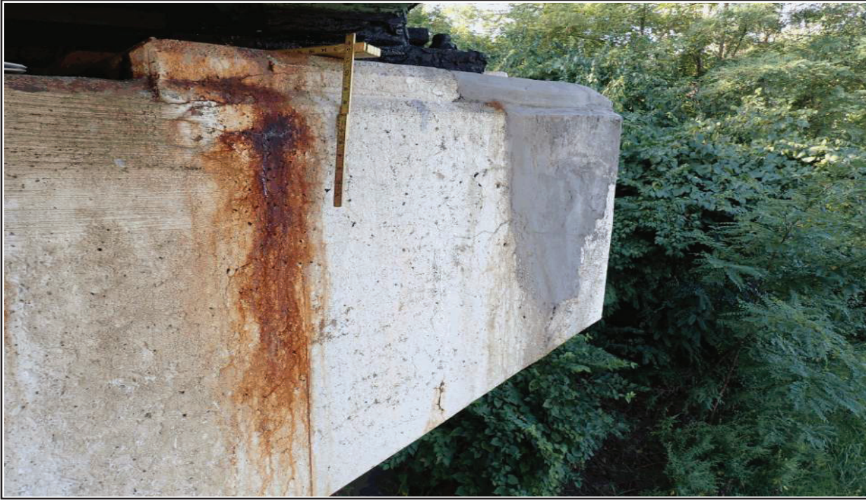
37 PIER 1, NORTH FACE, WEST END BELOW BEARING 1 - CRACKS WITH CORROSION STAINS
