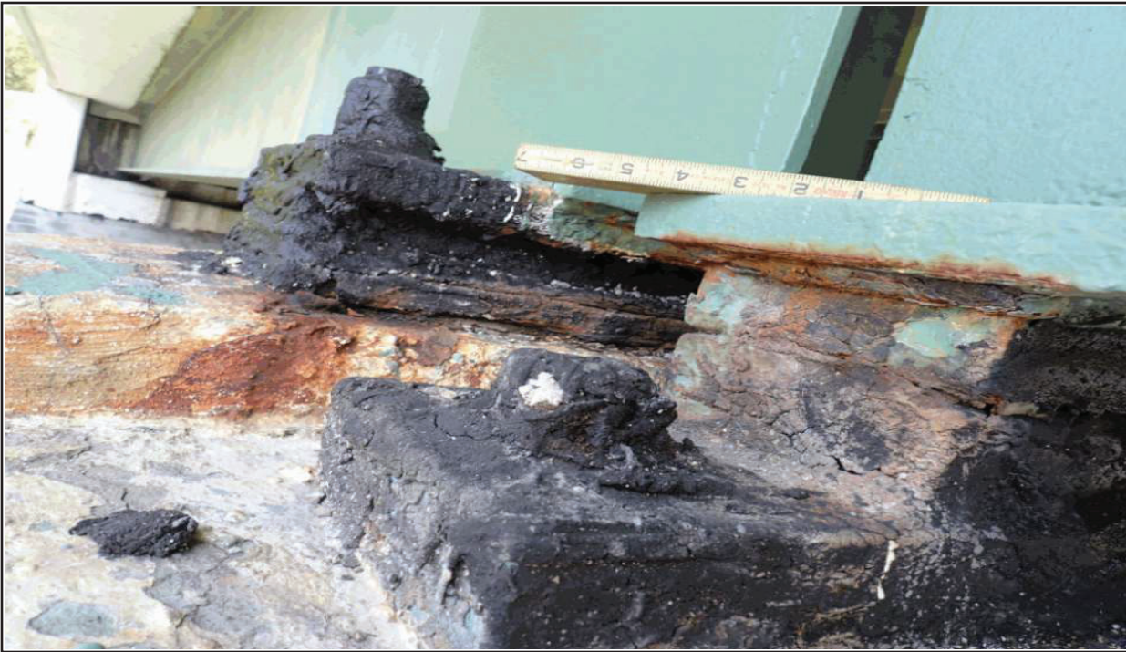
31 PIER 4, SPAN 5, BEARING 1 - LAMINAR CORROSION WITH SECTION LOSS ALONG MASONRY PLATE
