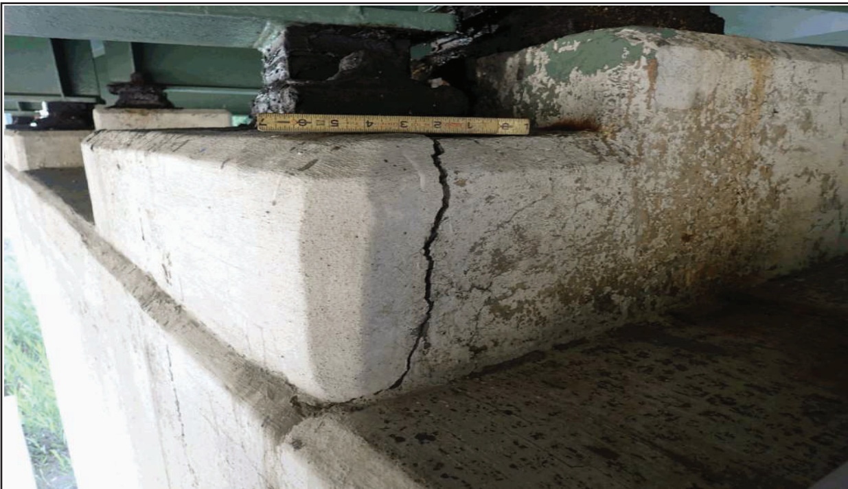
38 PIER 1, SPAN 2, PEDESTAL 3, NORTHWEST CORNER CRACK AND NORTH FACE DELAMINATION
