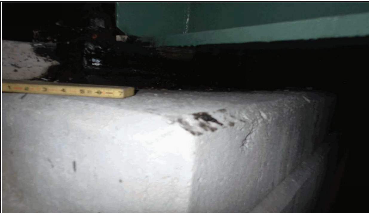
28 SPAN 2, PIER 2, BEARING 4 - COVERED IN GREASE (TYPICAL OF ALL)
