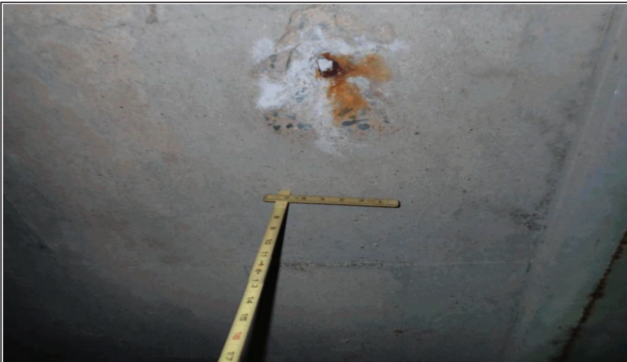
18 SOFFIT, SPAN 2, BAY 1 OVER THE LEFT LANE - SPALL WITH EXPOSED CORRODED STEEL REINFORCEMENT
