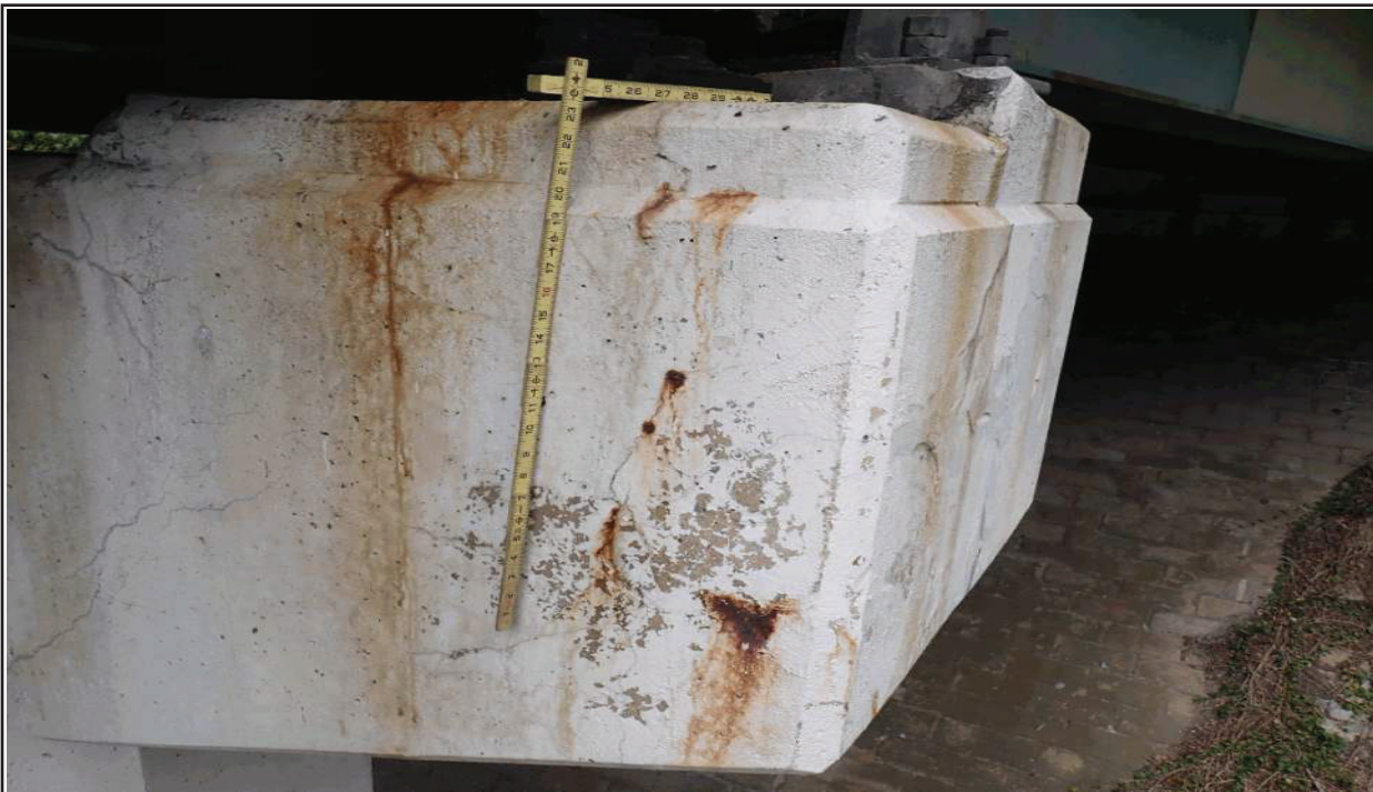
42 SPAN 4, PIER 4, SOUTH FACE BELOW BEARING 5 - CRACKS WITH CORROSION STAINS
