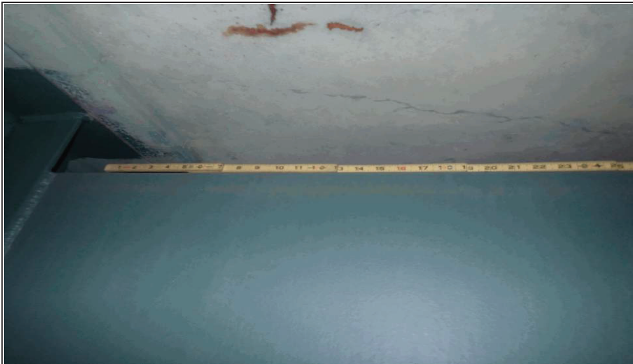
22 SOFFIT, SPAN 3, BAY 1 AT INTERIOR DIAPHRAGM 1 - CRACKS WITH CORROSION STAINS
