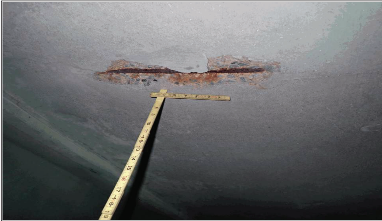
21 SOFFIT, SPAN 2, BAY 4 SOUTH OF PIER 2 - SPALL WITH EXPOSED CORRODED STEEL REINFORCEMENT WITH SECTION LOSS
