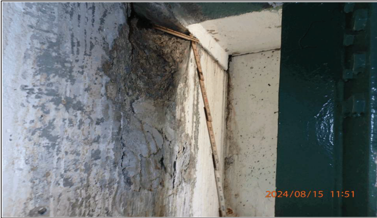
33 SOUTH ABUTMENT BACKWALL BEHIND GIRDER 1 - SPALL
