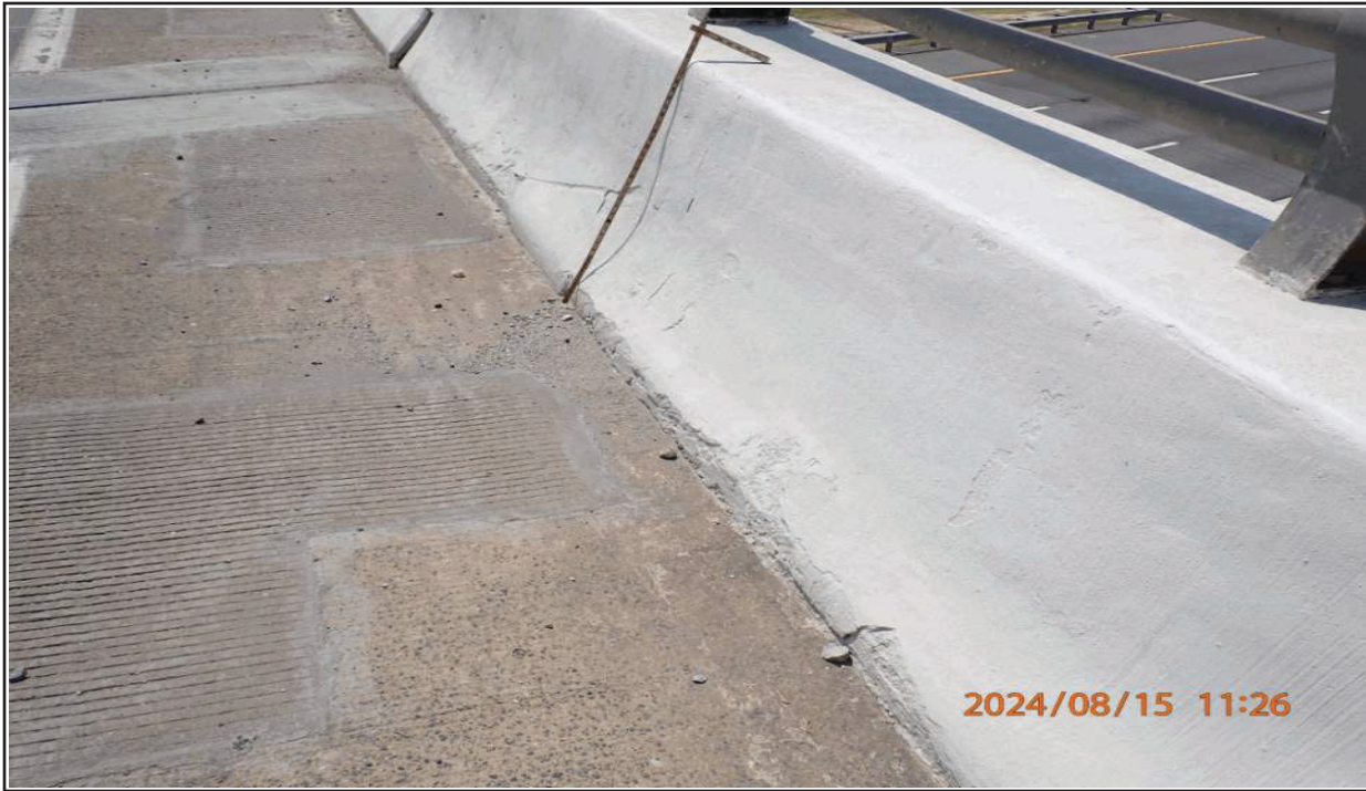
15 SPAN 5, WEST CONCRETE RAIL ALONG THE BASE - PAINTED OVER SPALLS
